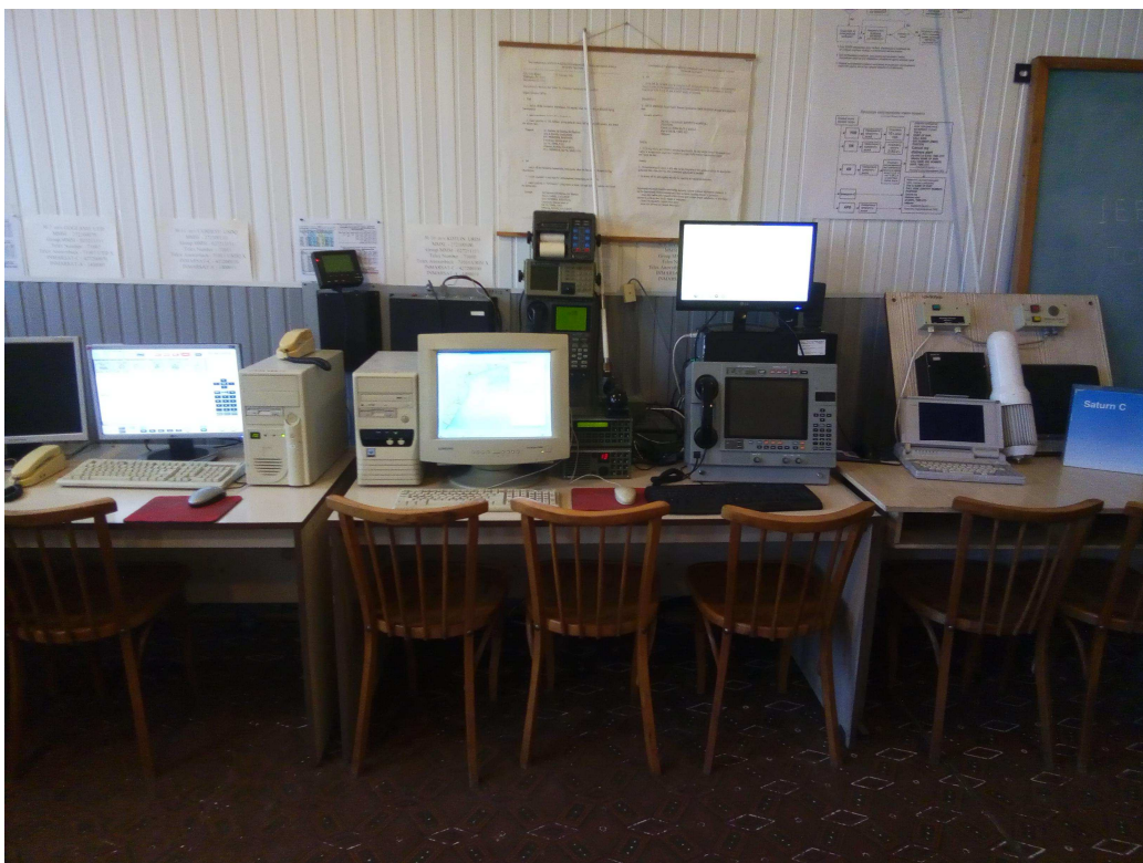
Picture 2. JRC real equipment, Integrated Radio Communication System, Inmarsat-C, AIS+ECDIS installation
